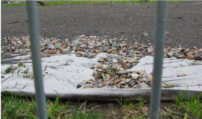
Figure 2: Geotextile fabric laid between natural ground and the road base reduces the amount of road base required, and the underlying soil profile is not disturbed or contaminated
