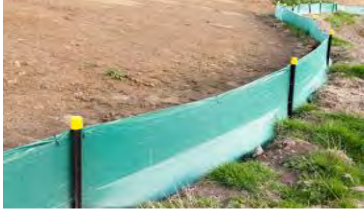
Figure 4: Woven sediment fence at lowest lying boundary to prevent sediment run-off from site.
